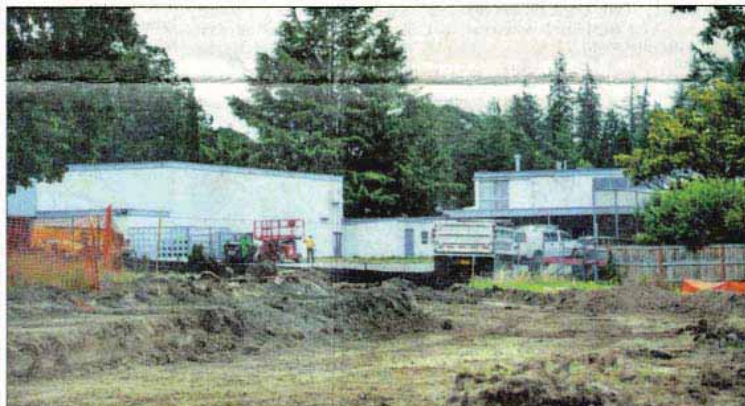
An access road cutting through Cedar Hills Park to William Walker Elementary is being made to assist with construction traffic during the renovations for both properties.
